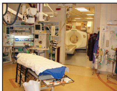
Figure 8: Direct access from trauma welcome area to a 64-slice CT scanner. On the other side there is direct access to an operation theater (not showing in the photo).
